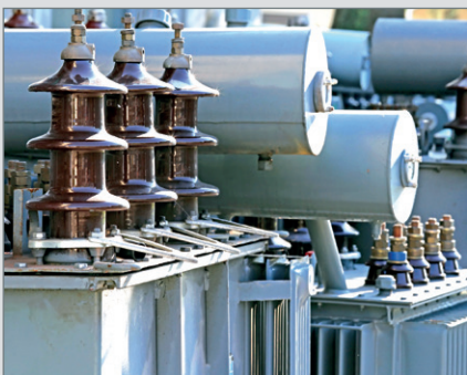
Power Generation: Noise and vibration are reduced on transformers and substation equipment
